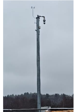
Closed Circuit Television (CCTV) for Traffic Monitoring.
