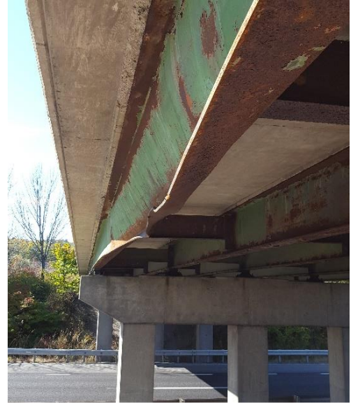
Exit 109 Interchange Bridge Damage in Augusta
